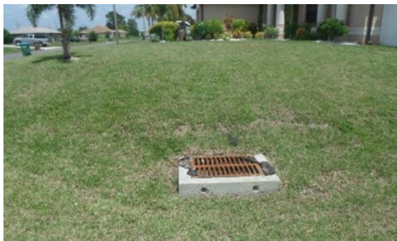
Raised Grate Inlet
