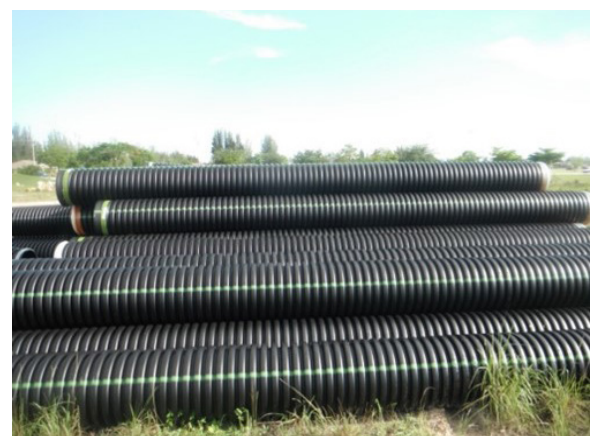
Stormwater Pipes (Black Color Pipes)
