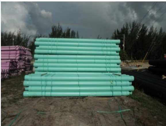
Sewer Pipes (Green Color Pipes)
