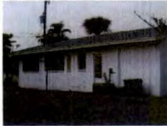
Area 6 – Residential Deterioration
