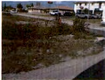
Area 9 – Neglected Infrastructure
